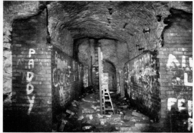
A ventilation shaft in the Bidston shelter which also doubled as an emergency exit
